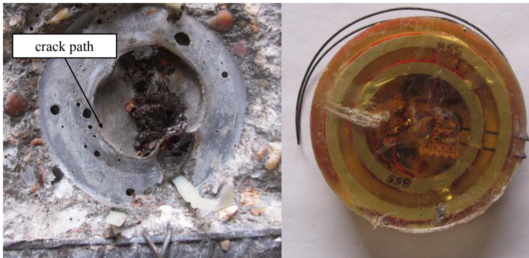
Figure 4-35 Crack Path Failing to Intersect Sensing Wire of B55 but Causing Corrosion of Reinforcement
