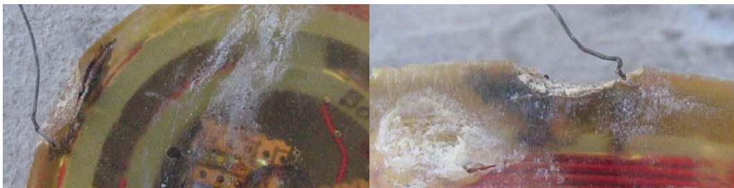
Figure 6-13 Black Corrosion in B04
