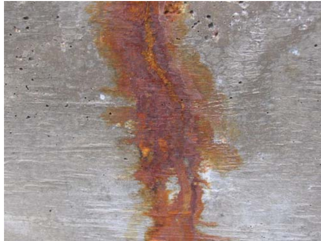
Figure 5-34 External Corrosion on the North Face of Slab 4
